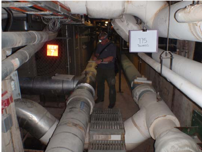
East Tunnel Intersection to Mall - PAT to Left, JFK in Front, TAW Beyond
