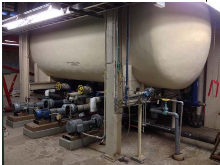
Rozell Central Plant - Hot Well Condensate Tank & Transfer Pumps
