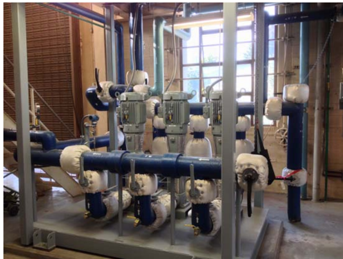
Rozell Central Plant - DA Boiler Feedwater Pumps
