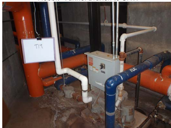
Typical Tunnel Electric Condensate Pump
