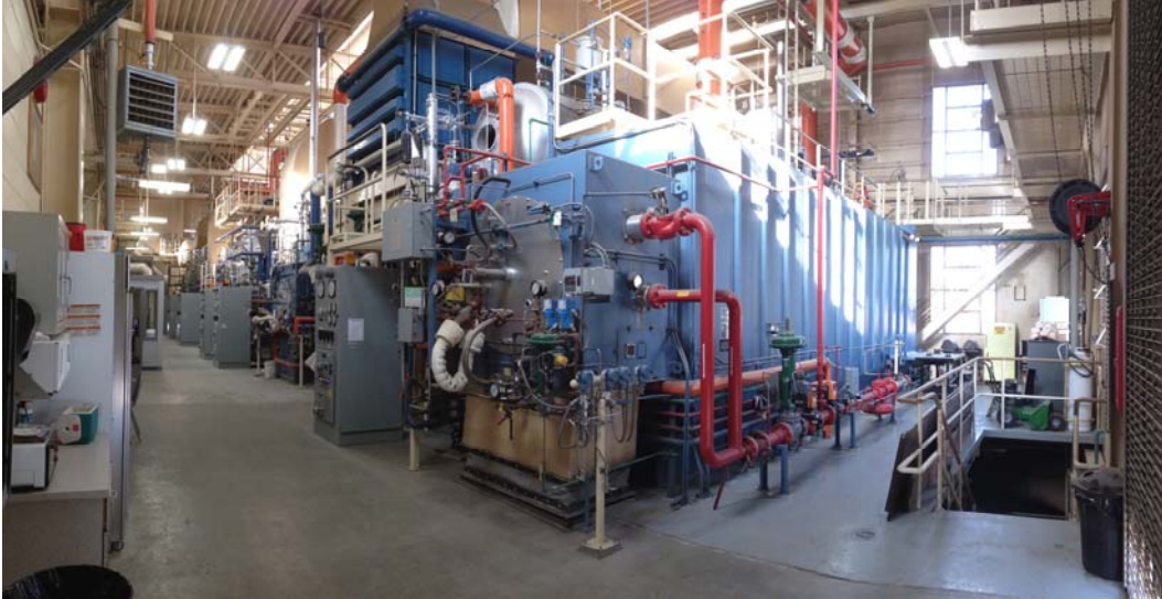
Rozell Central Plant - HP Steam Boilers
