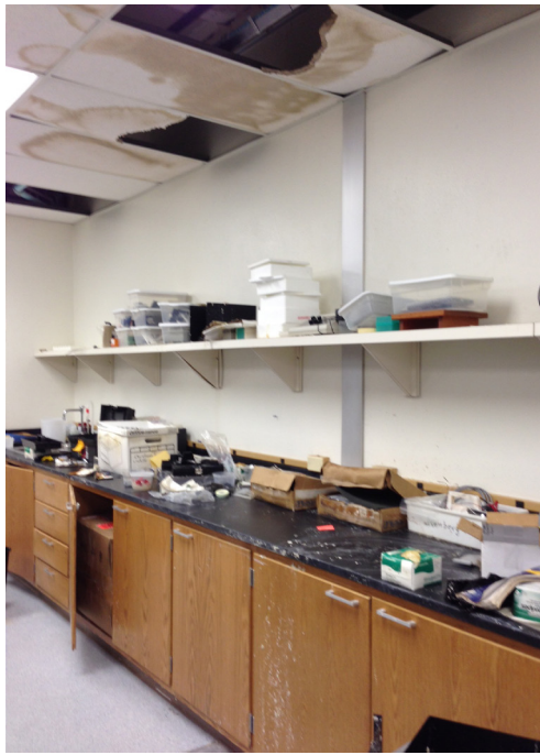
Figure 2.c EWU Science Building Water Damage
